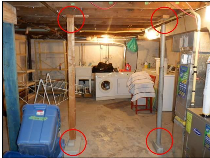
Poorly secured at top or bottom
