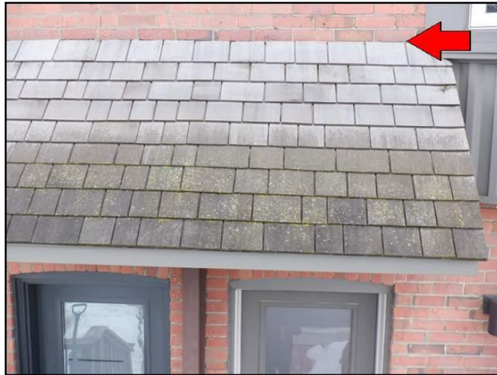
Flashing not visible...
